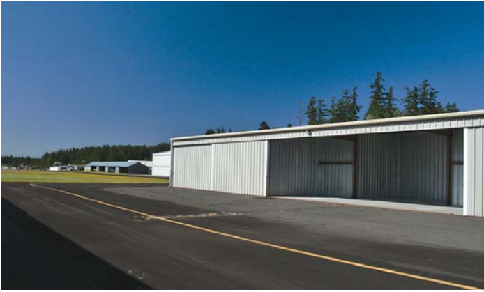
HANGAR AT FRIDAY HARBOR AIRPORT. 984± sq ft, wing section: 41'x16', tail section: 20'6" x 16'. NO sewer or water. Subject to an "Assignment of Lease" for the land under the improvement which is owned by The Port of FH. #412903 $75,000 www.SamBuck.com
